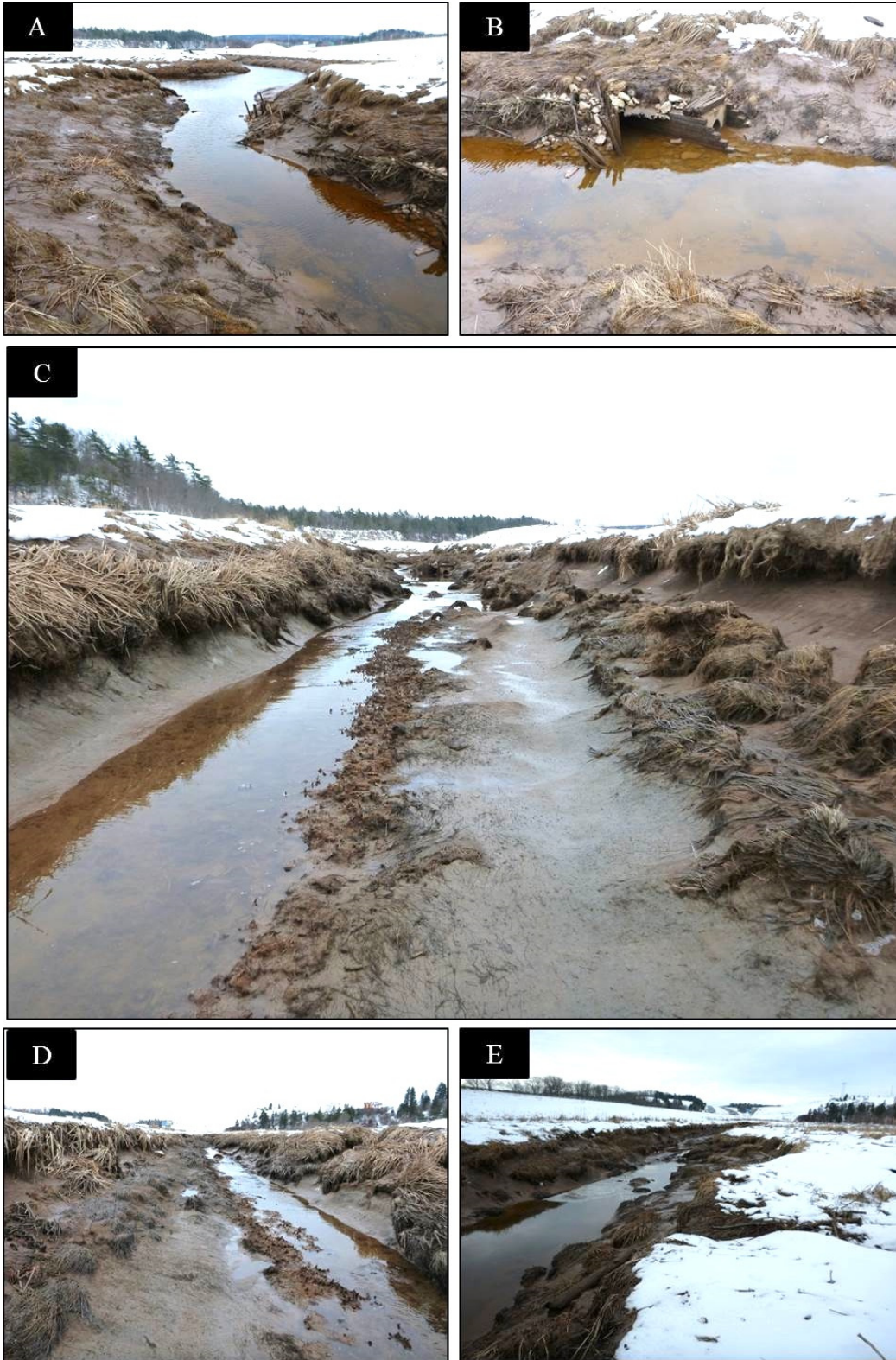
Figure 44 Main channel at SCW showing a) mouth of channel; b) old aboiteau structure; c) the scour and erosion along the right of the channel facing the River; and c) channel towards upstream; d) scour erosion and area where channel is now, continuing to erode back and deepen. Photographs by CBWES Inc., 21 February 2014.
